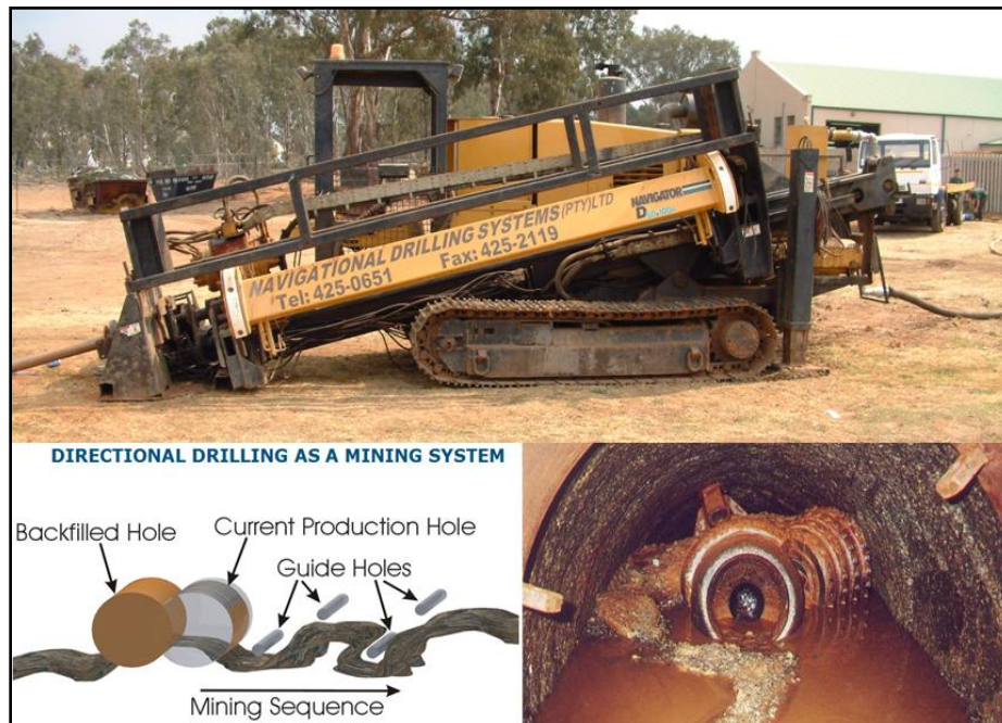
Illustration 3: Directional drill rig; insets showing reaming of pilot hole (bottom right) and ore extraction method (bottom left).
