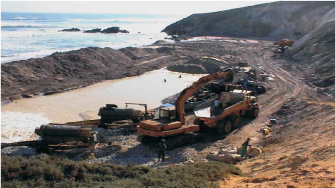
Illustration 8: Medium-scale beach mining operation using heavy machinery for gravel extraction and a central processing area.
