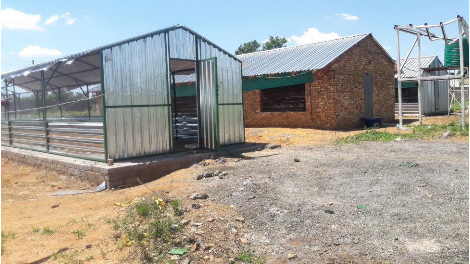
Figure 7. Examples of the houses built with iron sheets and another with bricks.
