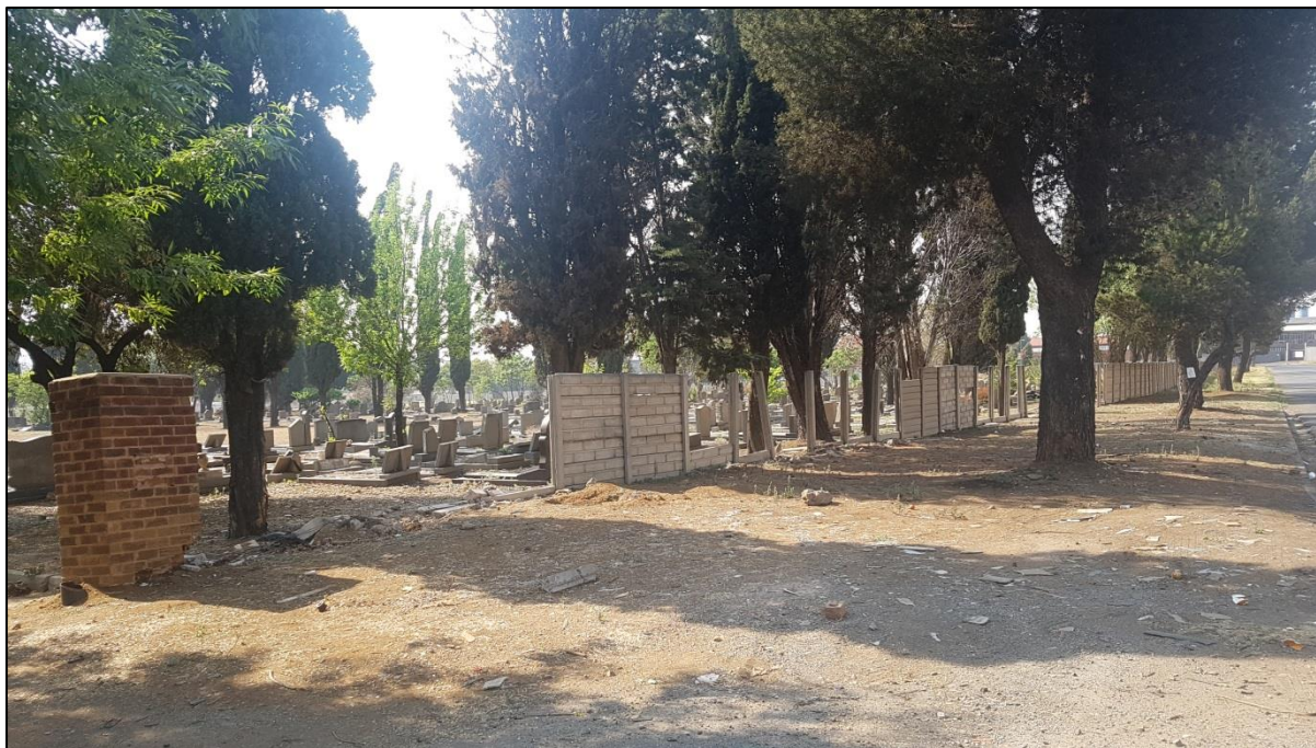
Figure 10 – View of partially destroyed wall on the north-western edge of the cemetery
