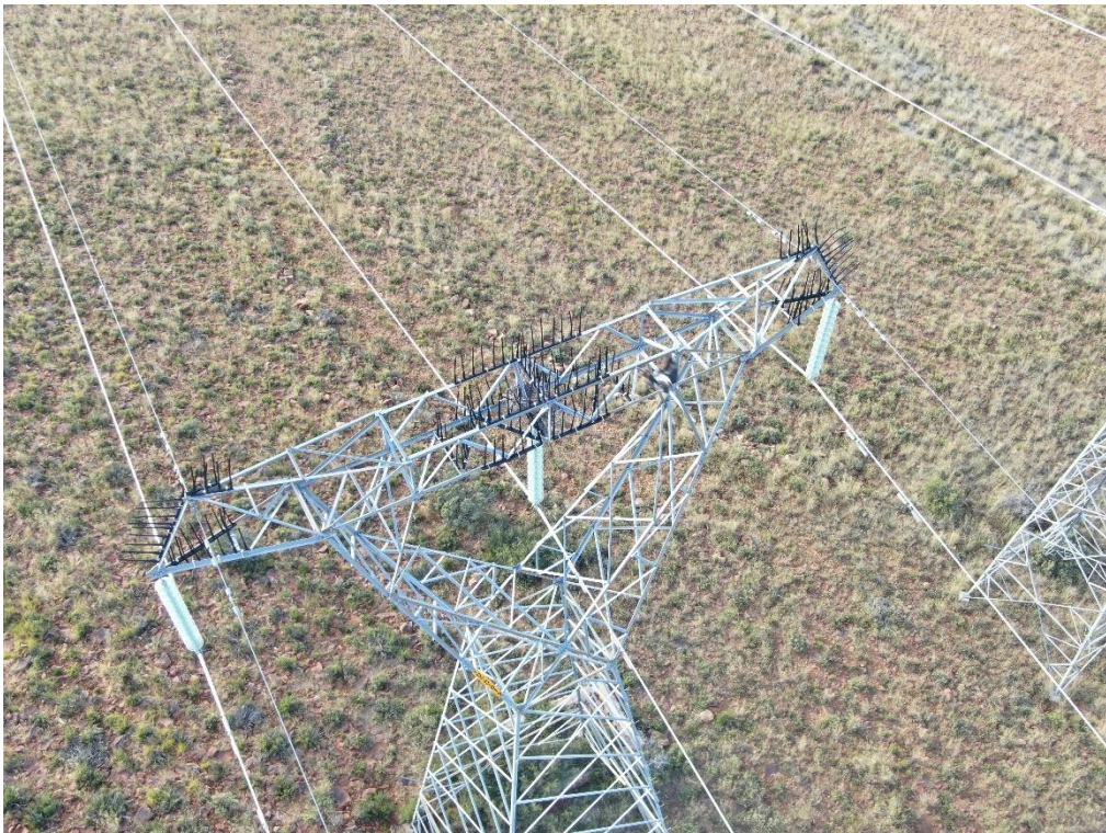
Figure 4: High voltage powerlines running through the PAOI.
