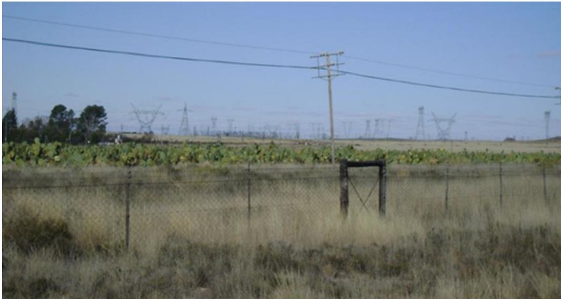
Figure 8: Power line infrastructure along the N10 national road.
