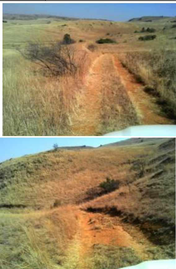
Figure 32: Surface cross drain (interventions W42C-02-221-00 to W42C-02-226-00) looking in a south and south-easterly direction
