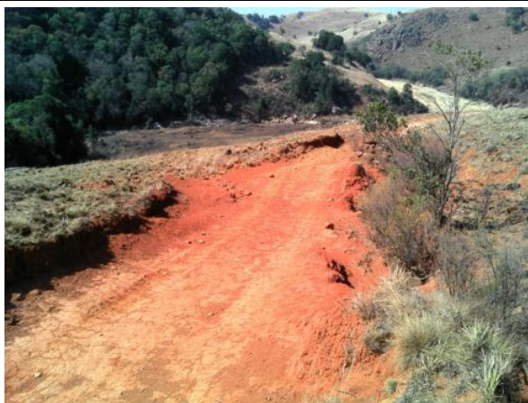
Figure 25: Road to be stabilised by surface cross drain (intervention W42C-02-213-00) looking in a south-easterly direction
