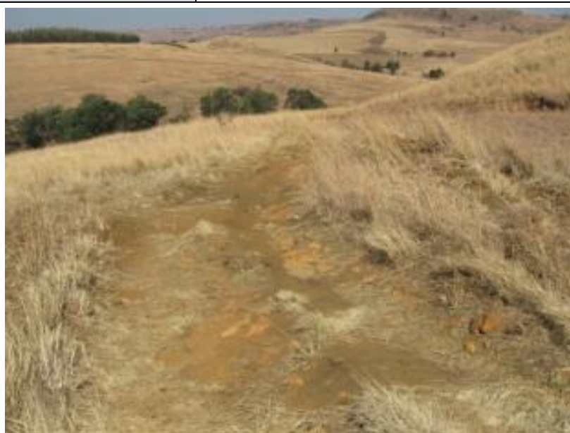
Figure 30: Section of road requiring concrete strips and adjacent trench (right side of road) to be backfilled (W42C-02-218-00), looking in a south-south-eastern direction
