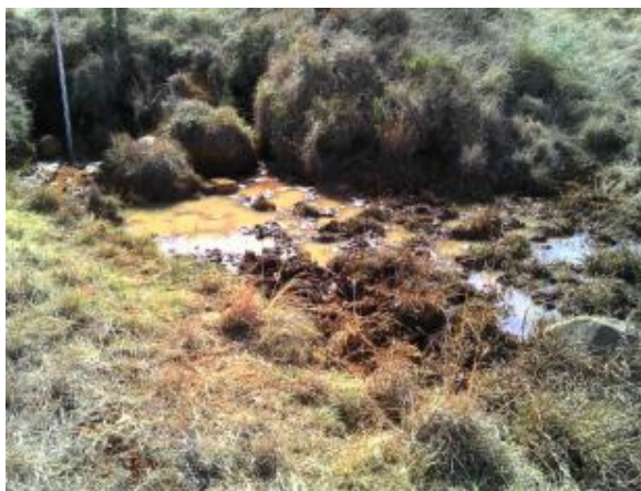
Figure 31: Headcut erosion stabilisation with concrete (intervention W42C-02-219-00) looking in a north-westerly direction
