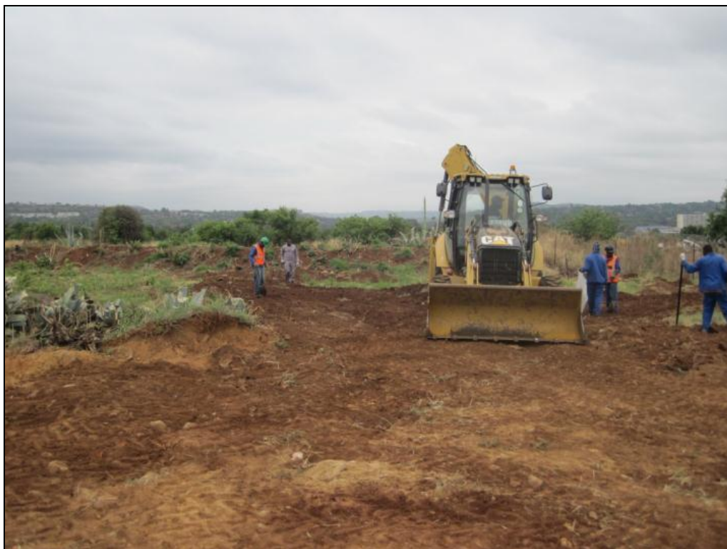
Figure 9. TLB used for grading down the soil heaps left over from the construction.
