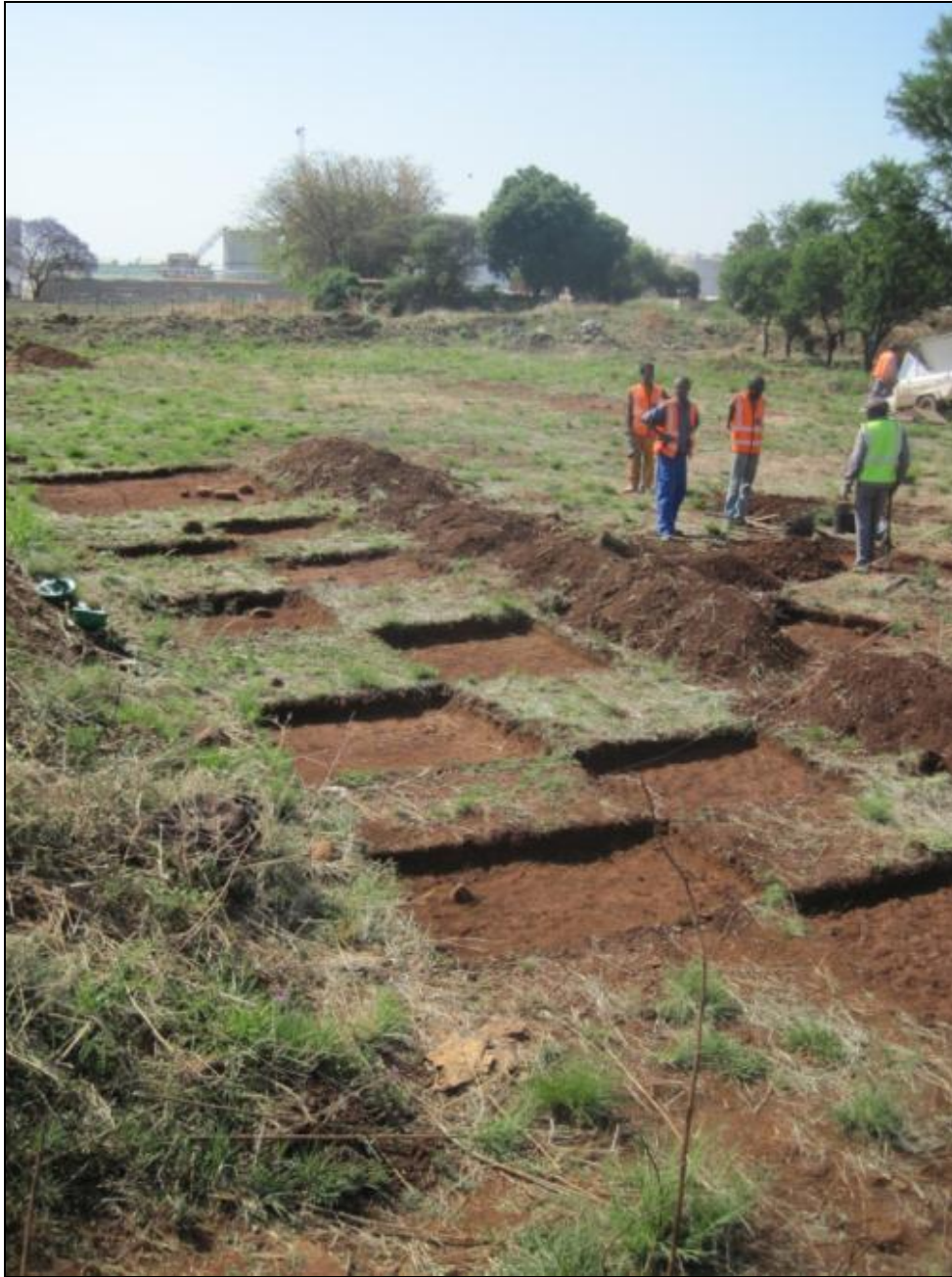
Figure 6 - 1m x 1m test excavation pits. Alternating test pits were excavated within the blocks to ensure maximum coverage.
