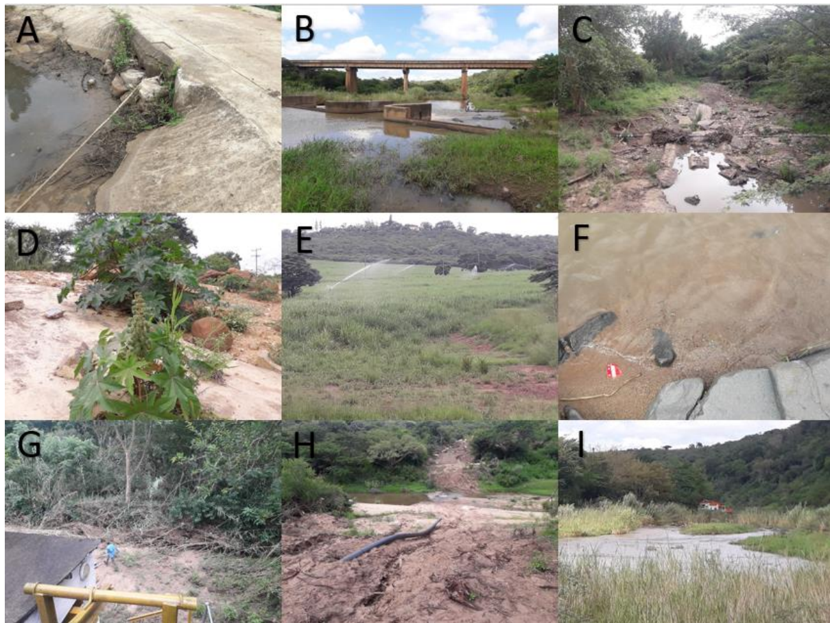
Figure 15: The impacts on the wetland’s health of the Mpungose WSS project area, A) Damming, B) Crossing structures and weirs, C) Eroded channels, D) Alien vegetation, E) irrigation, F) Sedimentation of systems, G) Water abstraction works, H) Pipeline installation and crossing activities, I Sand mining.
