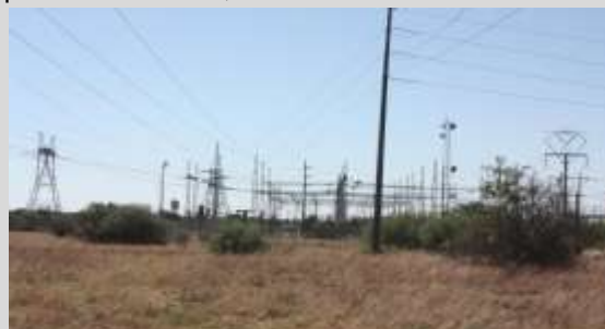
Figure 2: View of existing infrastructure within and around the Watershed Substation (study area) (Aken. 2014)
