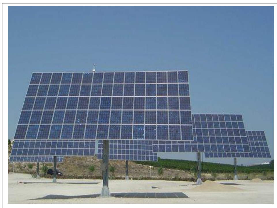
Figure 2.3: The support structures elevate the panels and allow for single axis tracking of the sun for increased efficiency (Source: energy blog)
