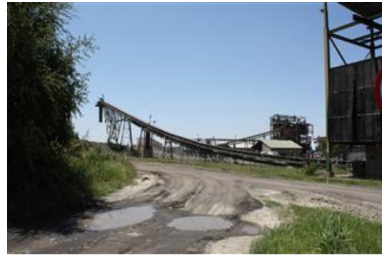
Plant and conveyor system
