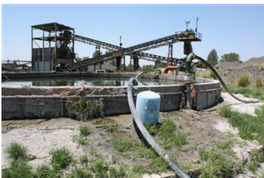
Water management infrastructure at plant
