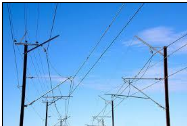
Figure 6: Example of an OHTE system
