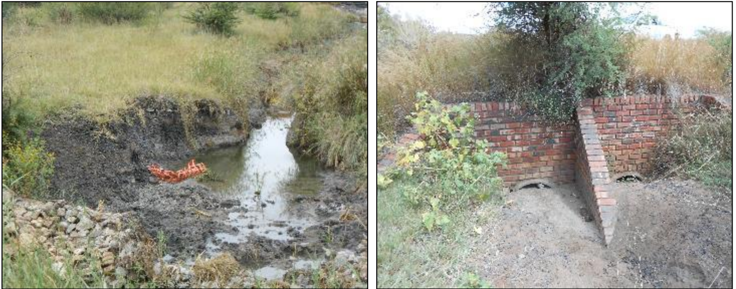
Figure 68: Erosion and Sedimentation evident at crossings within the RPM boundary.
