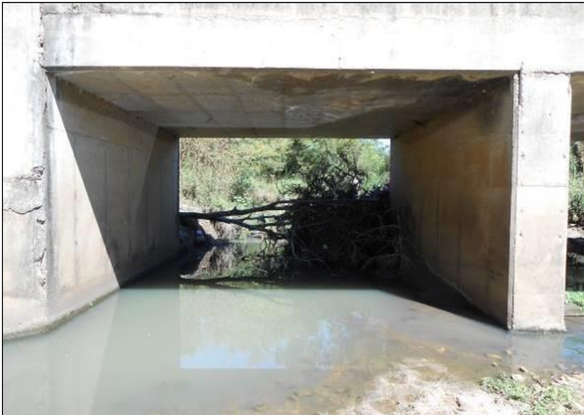
Figure 70: Blockages present at monitoring sites, restricting movement of debris downstream.
