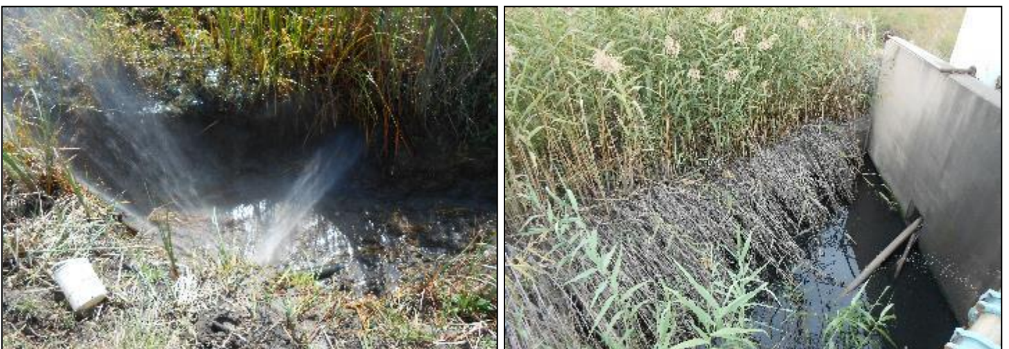
Figure 73: Leaking pipes within the RPM operations boundary.
