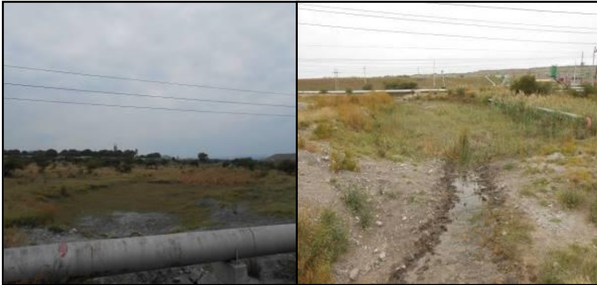
Figure 19: Erosion observed along the pipeline crossing within Klipgatspruit.
