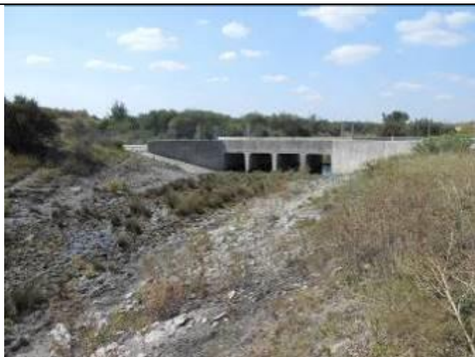
Figure 60: Upstream view of the SASS 40E located on the Hoedspruit. The site was dry at the time of the assessment.
