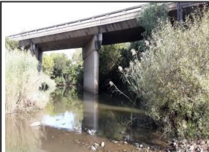
Figure 47: Upstream view of the SASS 22 site indicating the low flow at the time of the assessment.
