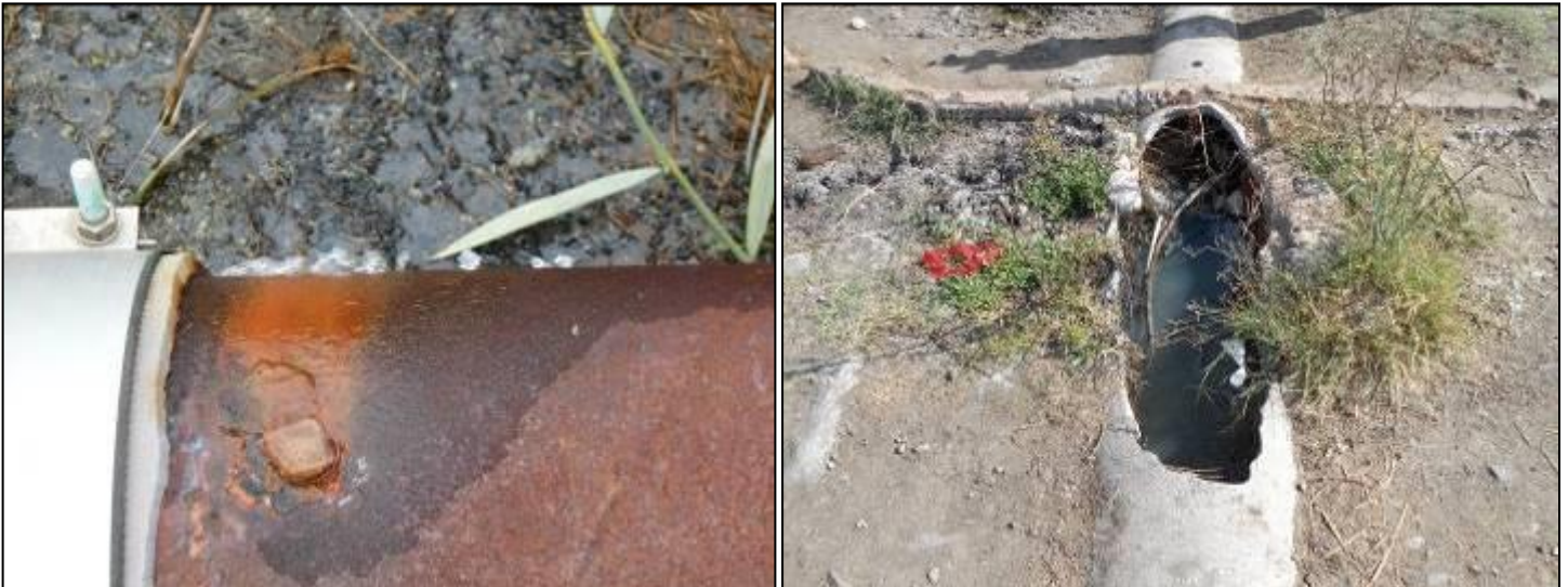
Figure 74: Leaking pipes within the RPM operations boundary and broken pipes within the rural residential area.
