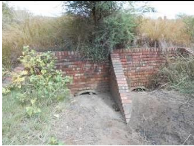
Figure 58: Upstream view of the SASS 35A site located on the Wildebeesfonteinspruit. The site was dry at the time of the assessment and culverts largely silted up.
