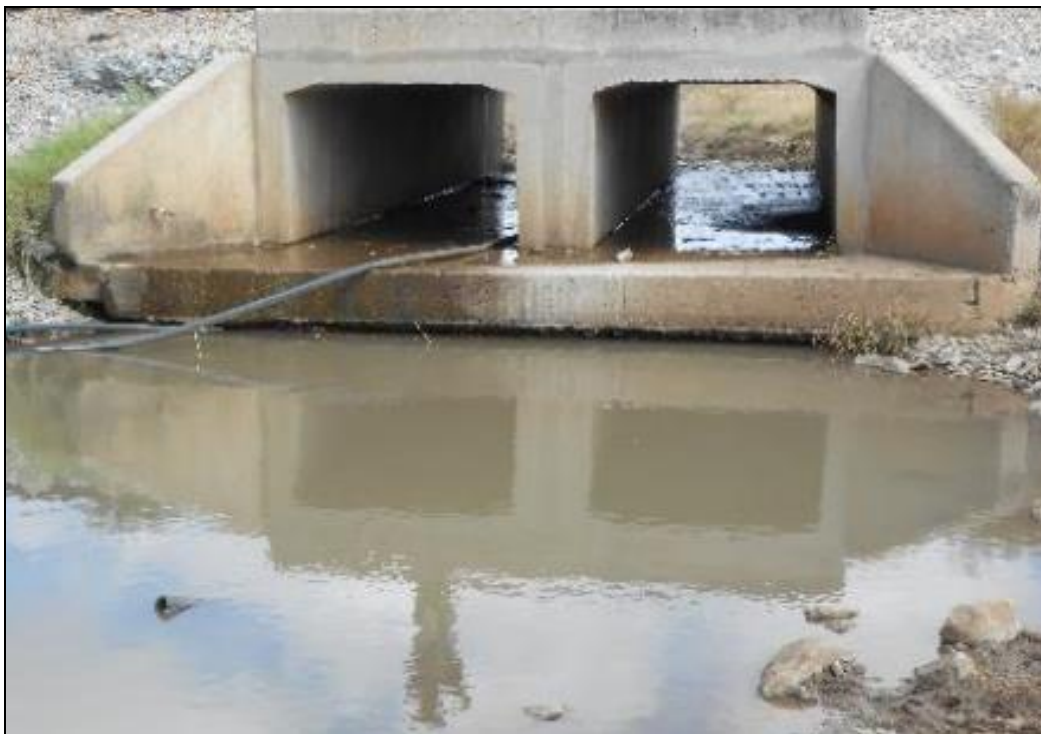
Figure 69: Culvert Bridge indicating the scouring and undermining of the Culvert structure resulting in altered stream hydrology.
