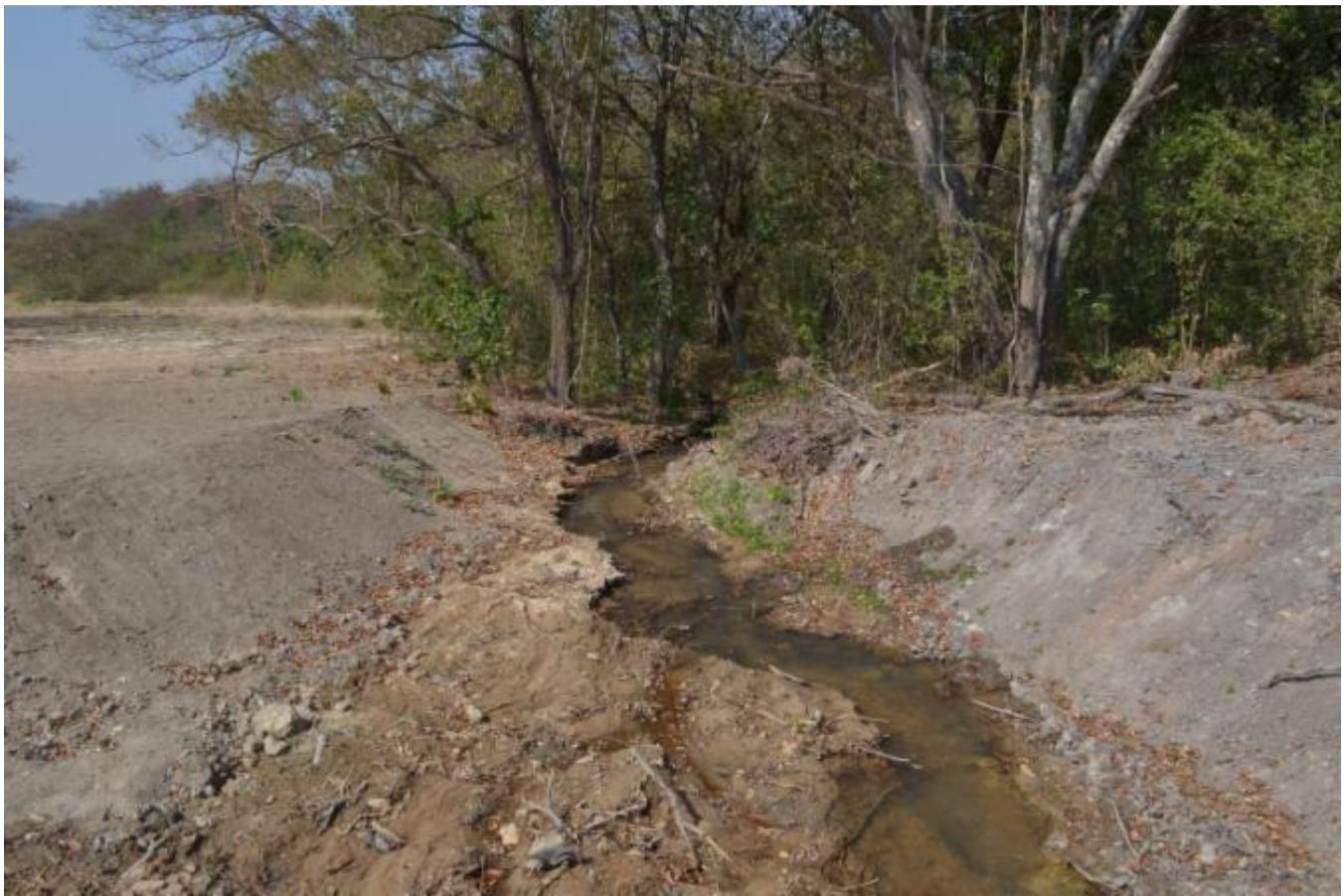
FIGURE 7 – EXAMPLE OF ROAD CONSTRUCTION ACTIVITIES THAT HAVE IMPACTED A WETLAND IN THE STUDY AREA NEAR THE EMNOTWENI CASINO COMPLEX
