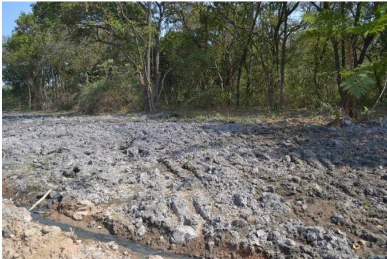
FIGURE 3 – HYDRIC SOILS EXPOSED BY ROAD CONSTRUCTION ACTIVITIES. NOTE THE WOODED RIPARIAN ZONE OCCURRING WITHIN THE WETLAND IN THE BACKGROUND
