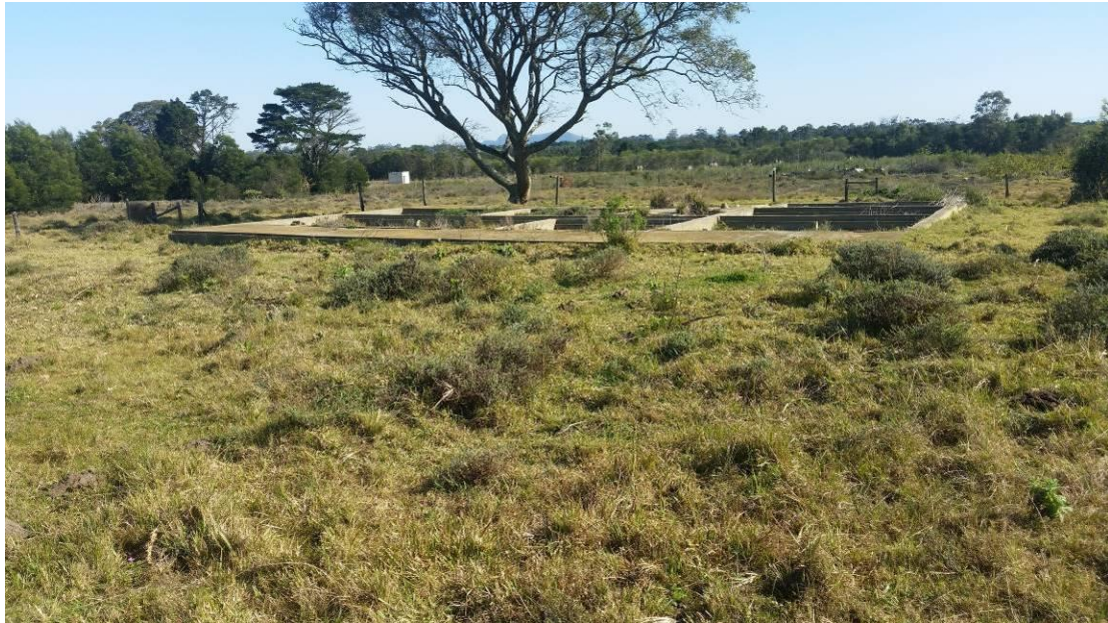
Figure 11: The old foundation ruins at Wetland 2. The wetland occurred between the ruins and the bush in the background.
