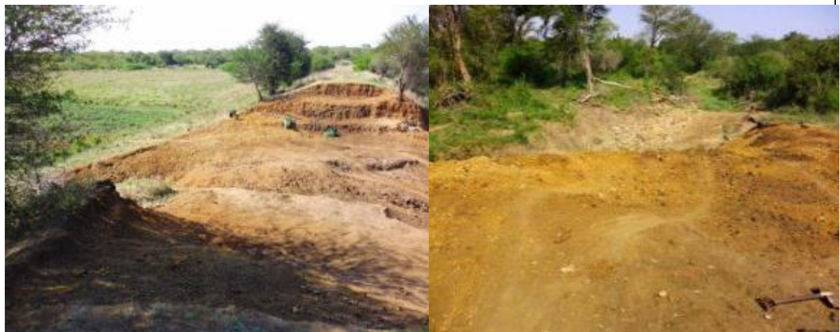
Picture showing the breach in the Silolweni Dam wall
