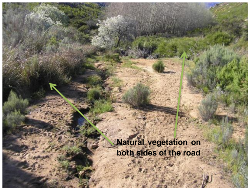
Figure 47: A photo of the road currently cutting through the Kraainfontein wetland (Courtesy: Donovan Kotze)
