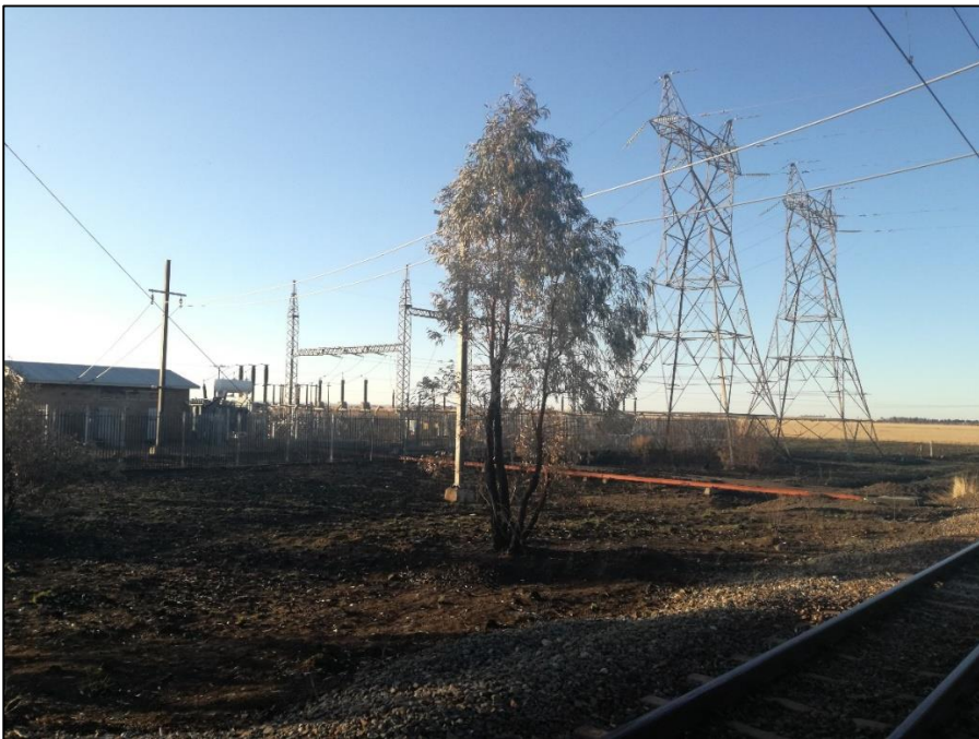
Figure 18: Power lines feeding into the Leeubos TR 132kV Traction Substation
