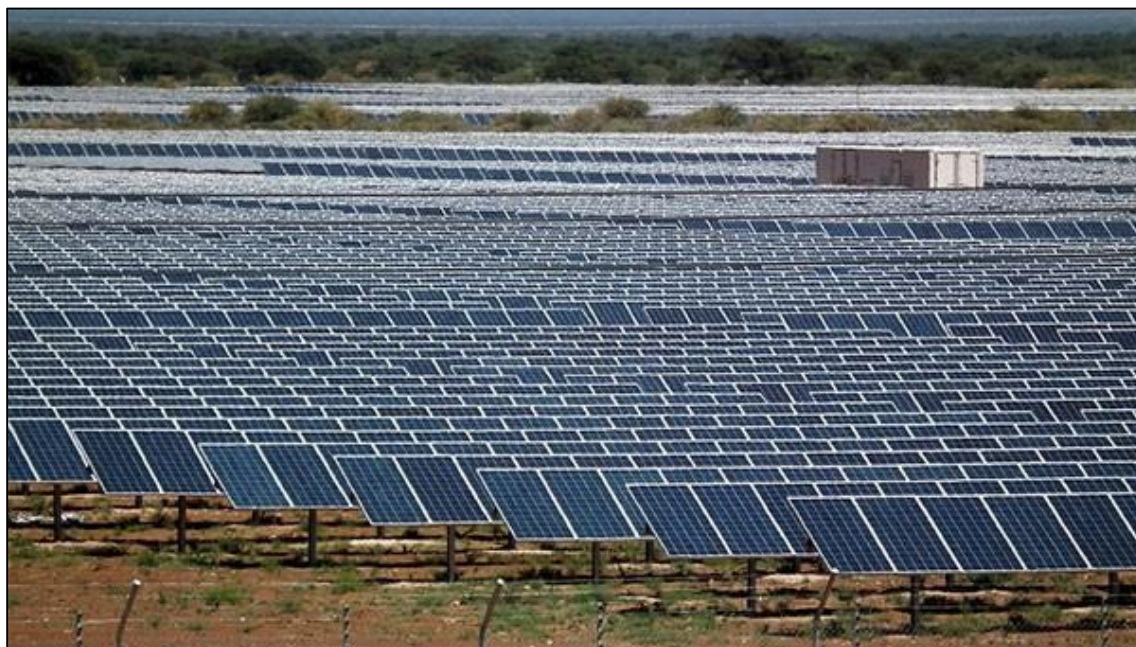
Figure 56: Kathu Solar Power Plant (photo courtesy of 'visits to the park'), near Kathu, Northern Cape Province
