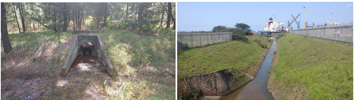
Photographs 5.4: Concrete culvert outlet from the artificial drainage channel linking into another channel within the greater drainage network (left); and the section of the artificial drainage channel exiting into the Richards Bay Port area (right).
