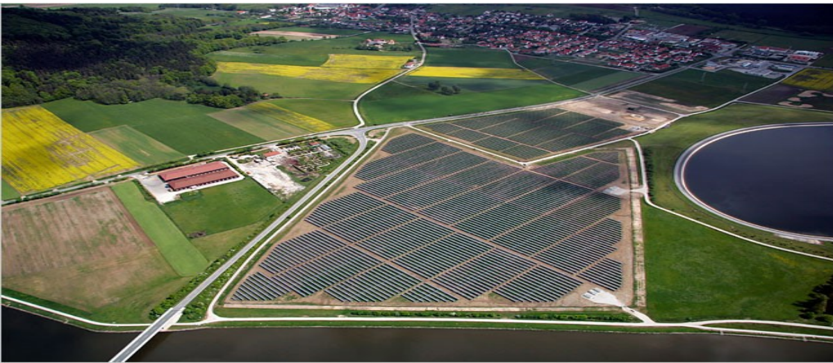
Figure 7. Aerial view of large scale Solar PV array
