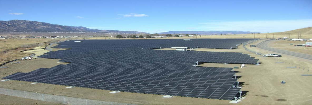
Figure 6. Large scale Solar PV array
