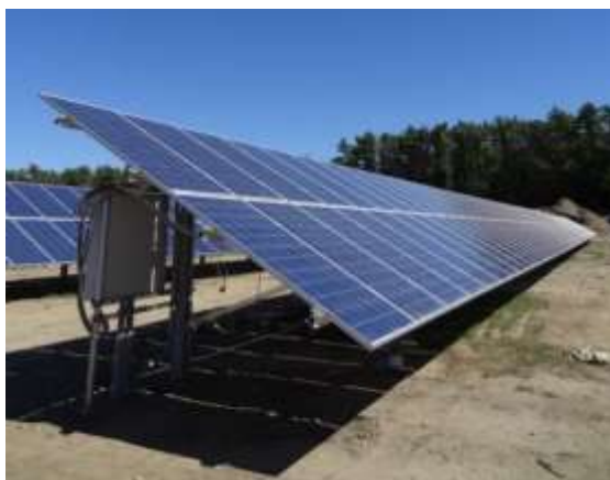
Figure 2: Photovoltaic panels (Photo courtesy of BlueWave Capital SA)
