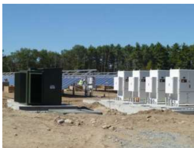
Figure 5: Inverter (Photo courtesy of BlueWave Capital SA)
