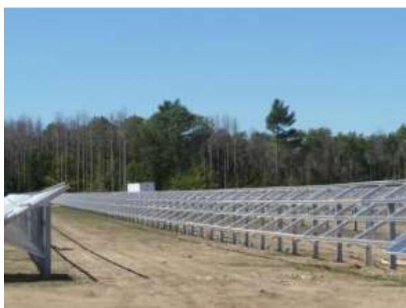
Figure 3: PV panel support structures (Photo courtesy of BlueWave Capital SA)
