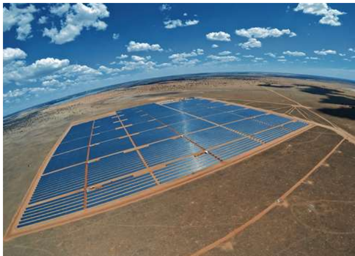
Figure 2.4: Photovoltaic (fixed-tilt/static) panel array (Photo: used with permission from Genesis Eco-energy Developments).
