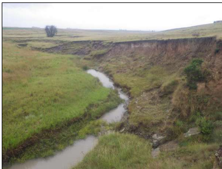
Figure 7-1: Erosion within the Klein Olifants River below Site KO2 (March 2016)
