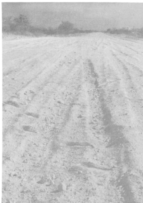
FIG. 2. Unsuccessful use of powder calcrete as gravel road material.
