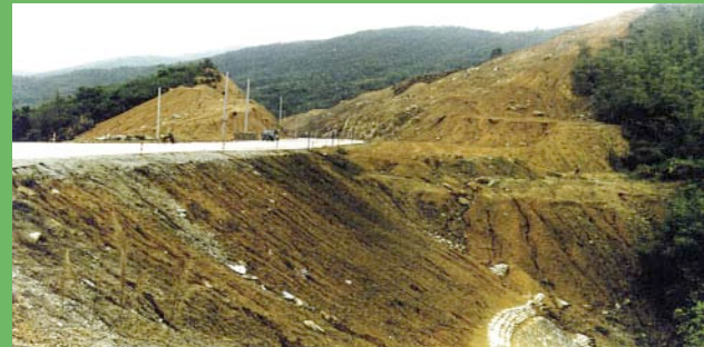
China - unstable highway fill prior to VS treatment. Road stability was so bad in untreated state that major lateral cracks in the pavement occurred
