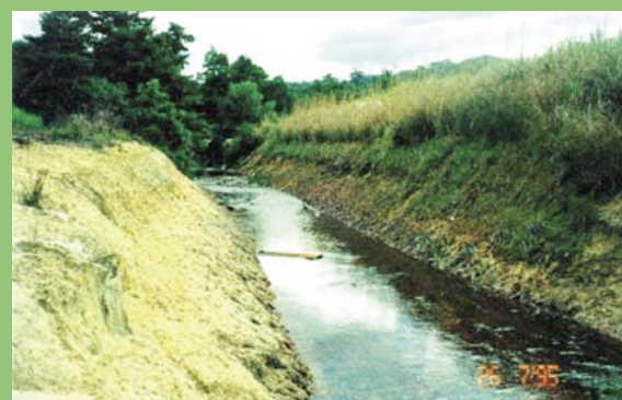
Australia - VS protects the right hand bank of a drain cut through acid sulphate soils of Queensland. Note left hand bank is devoid of any vegetation
