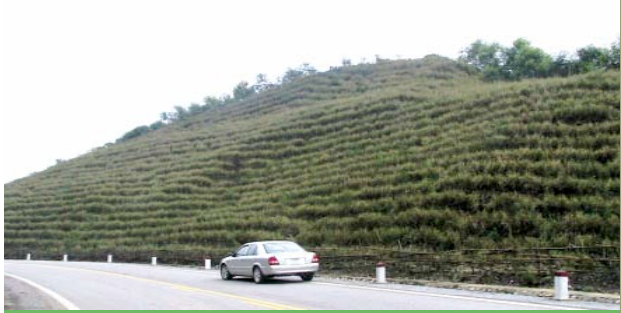
Vietnam: the Ho Chi Minh Highway has been stabilized with vetiver grass. The batters and fills are stable and withstand cyclonic rainfall events
