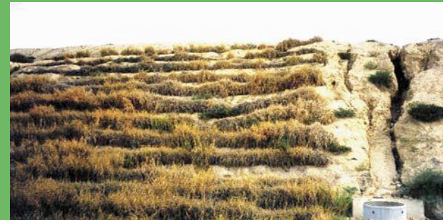
Spain - unstable and eroding highway fill treated with VS. Untreated eroded fill on right. VS grows well under low rainfall Mediterranean climate
