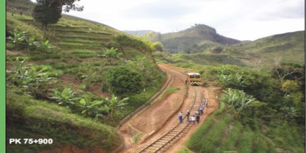
Disaster mitigation - this railroad in Madagascar was closed down by frequent cyclone damage. Stabilization with vetiver was vital in its rehabilitation
