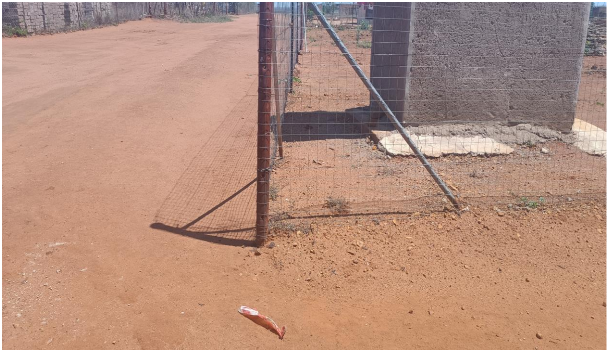
Shows the peg where the pole will be planted indicated by a danger tape
