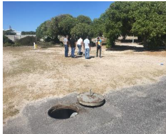
Existing WACS man hole on the front haul alignment
