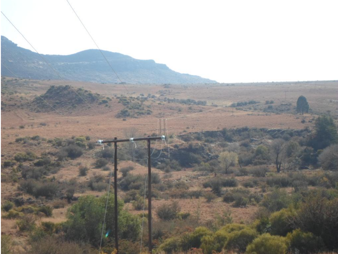
Image 2: Erosion gully along the route of the proposed line as observed from the top of the hill
