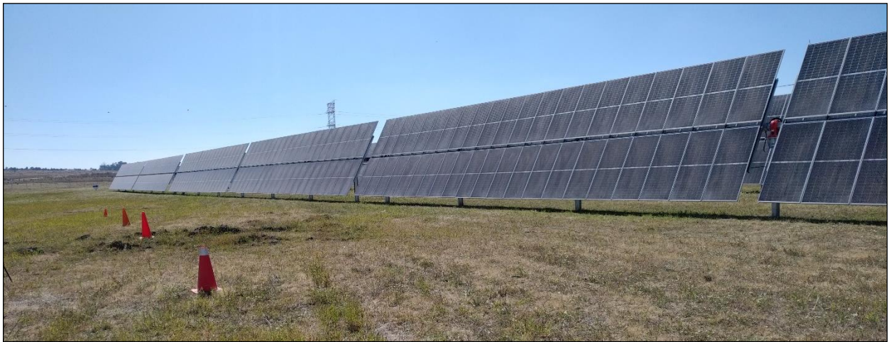
Figure 2 Frontal views of the PV arrays mounted on horizontal 1-axis tracker
