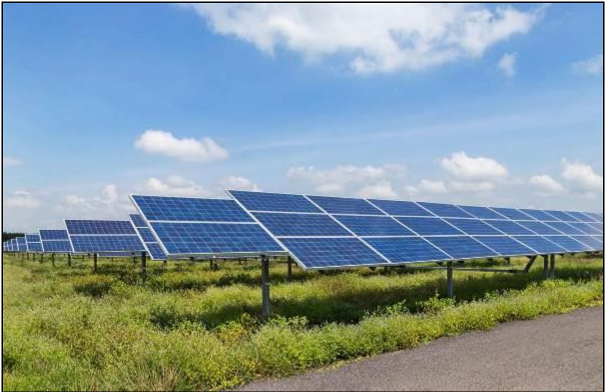
Photograph 1.1: Typical PV SEF facility
