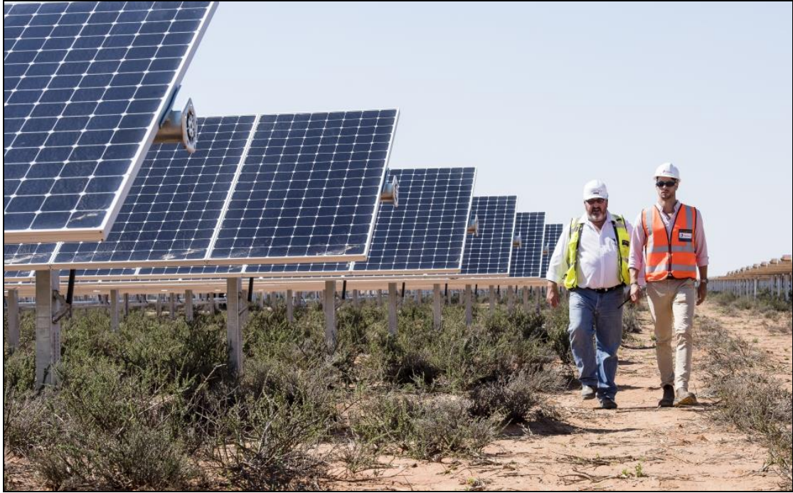
Figure 1: Photovoltaic (PV) solar panels. (Photo: SunPower Solar Power Plant-Prieska)
