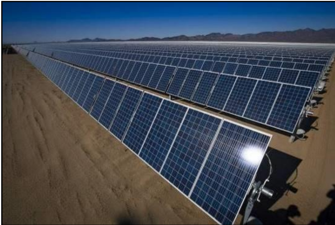
Photograph 1.1: Typical PV SEF facility
