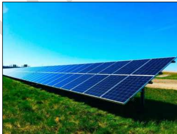
Figure 14 : Tilted Solar Panels with landscaped surface area
