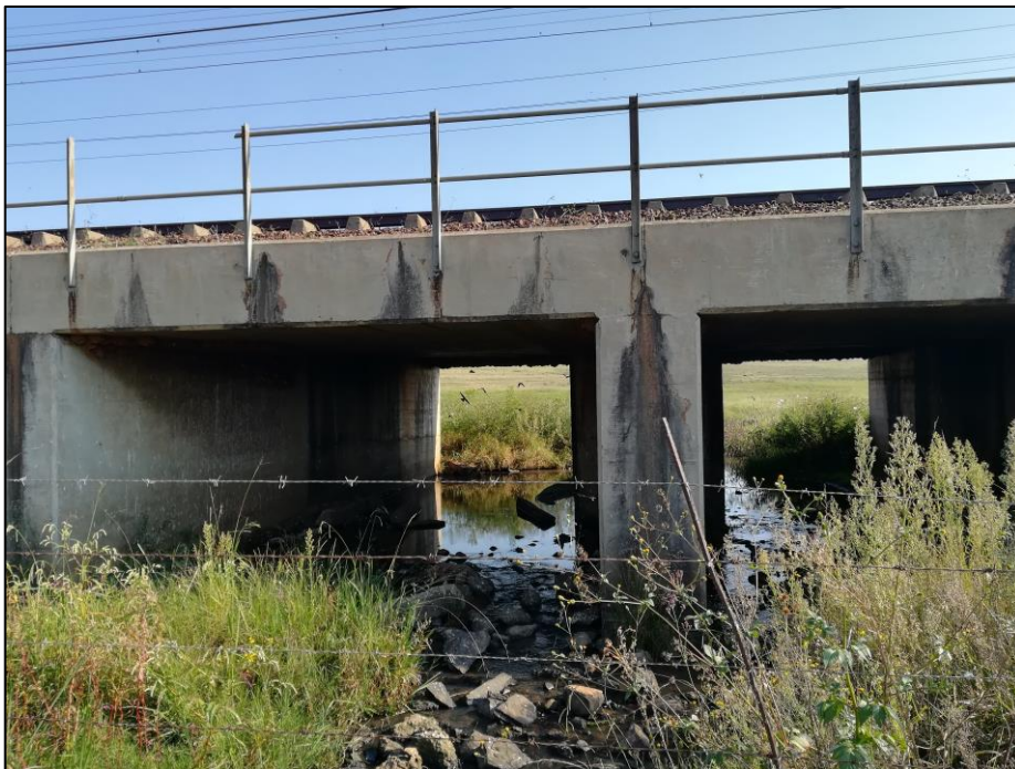
Figure 10: Railway bridge containing nests of a relative large colony of South African Cliff Swallow.
