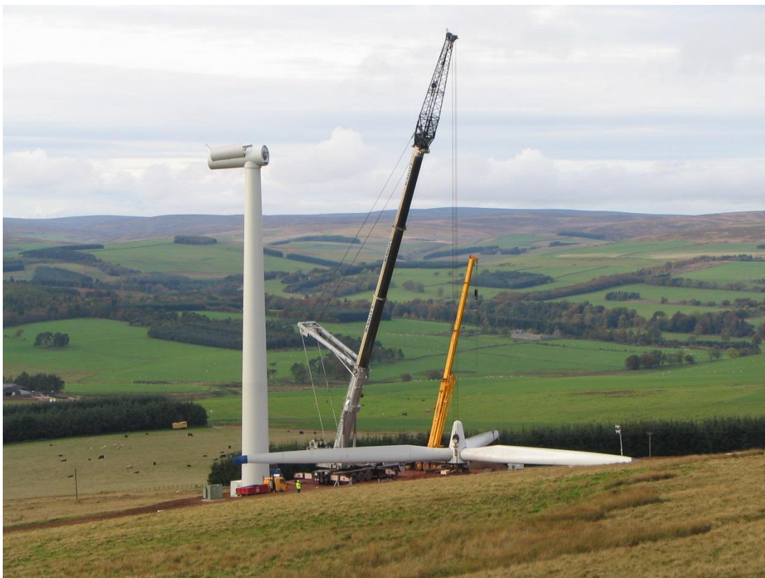
Example of a tower on which the rotor is mounted
