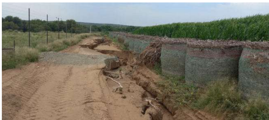
FIGURE 14: EROSION GULLIES AS A RESULT OF UNUSUAL HIGH RAINFALL
