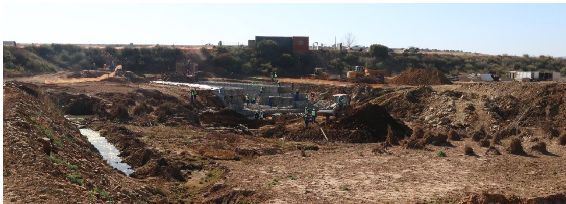
Figure 15: Construction adjacent to the river and within the floodplain and associated wetland areas clearly cause significant disturbance and impacts.
