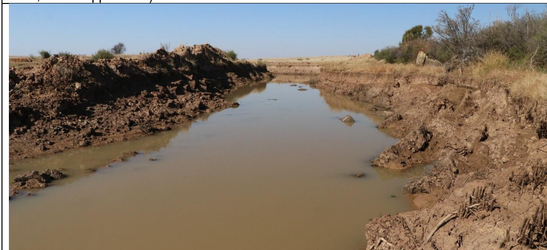
Another view of the main channel where the effect of sediment accumulation is also clearly visible.
