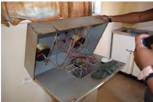
Figure 7 | Filter control console
