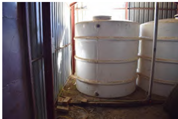
Figure 10 | Chemical storage tanks
