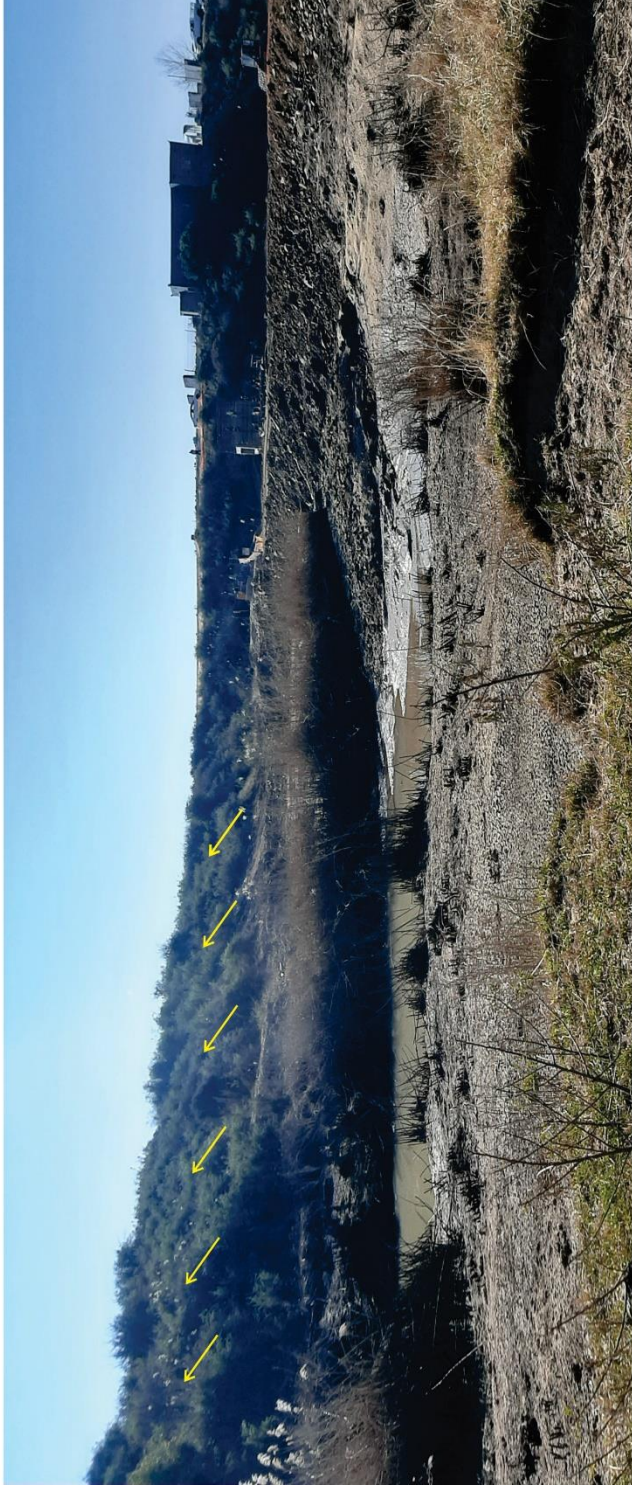
Figure 16. The concrete weir and an accompanying berm (below), looking west-southwest and east-northeast, respectively.
