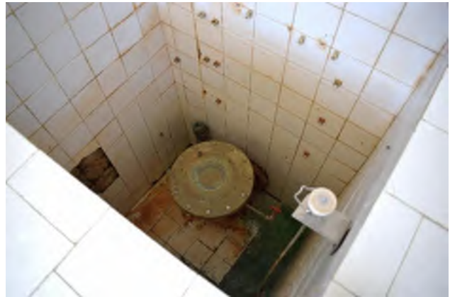
Figure 4 | Filter control weir and outlet valve (with missing tiles and hydraulic control pipework)
