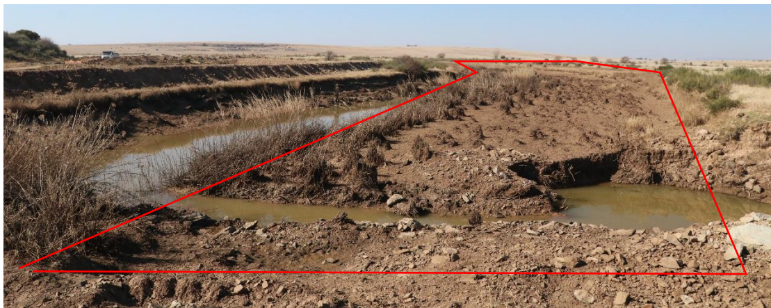
Figure 1: Portion of the Sandspruit proposed for dredging operations (red). Note current construction activities to the left of the site.
