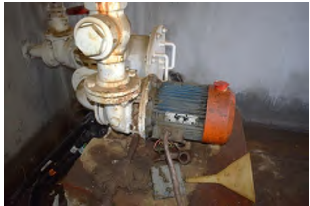
Figure 6 | Sedimentation tank jet pump
