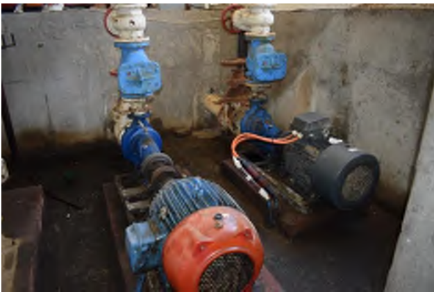
Figure 5 | Treated water pumps
