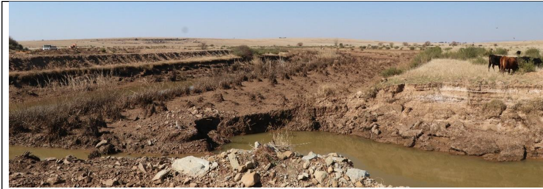
The eastern floodplain also contain extensive wetland areas though is currently also being affected by construction activities.
