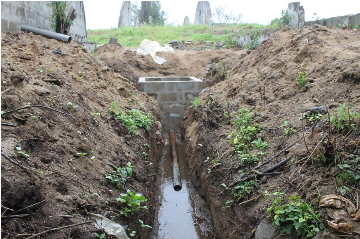
Figure 25. Image of excavation adjacent to existing hatchery operations. Not aeolian sands at depth within trench.
