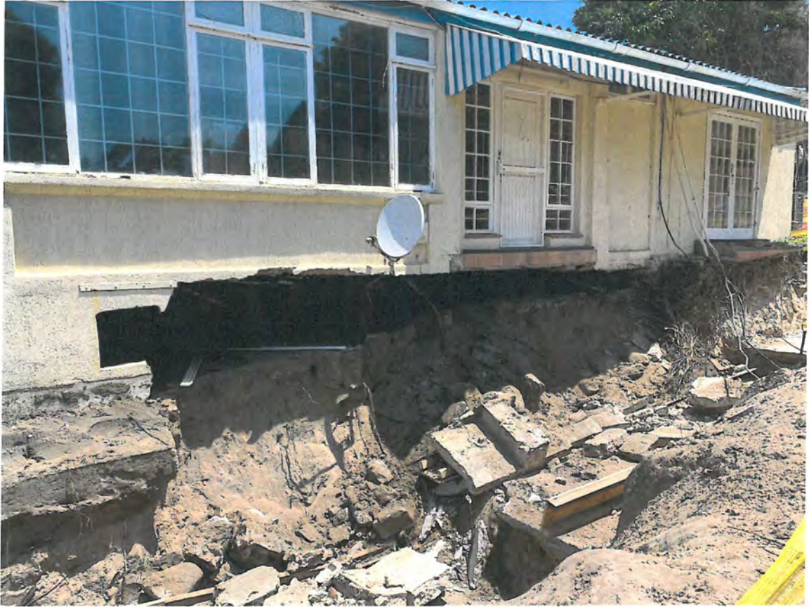
Damage to foundation wall on 5 November 2021
