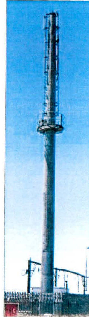
TYPICAL MONOPOLE MAST (UNPAINTED) GALVANISED
