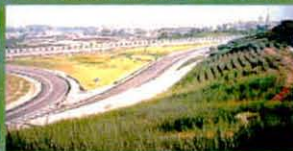
China - expressway stabilization. This cut was prone to massive slip. Stabilization with VS has given complete protection
