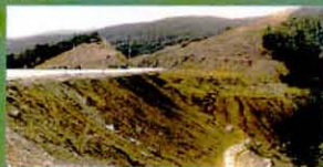
China - unstable highway fill prior to VS treatment. Road stability was so bad in untreated state that major lateral cracks in the pavement occurred
