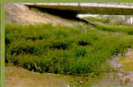
Australia - this river bank and bridge abutment have been stabilized with vetiver. Vetiver is an excellent interface for concrete and soil
