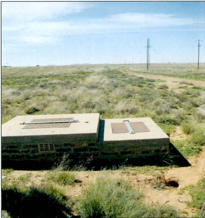
Fig.12 Water pipeline at Knapdaar 14, Springfontein.
