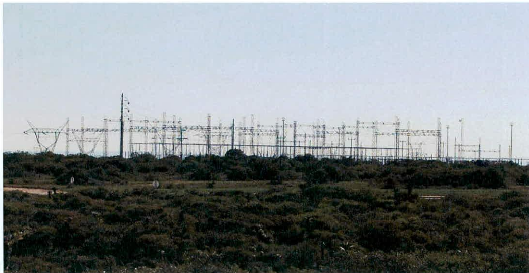
Figure 3.3 Substation just north of the wind turbine site (approximately 500m away).
