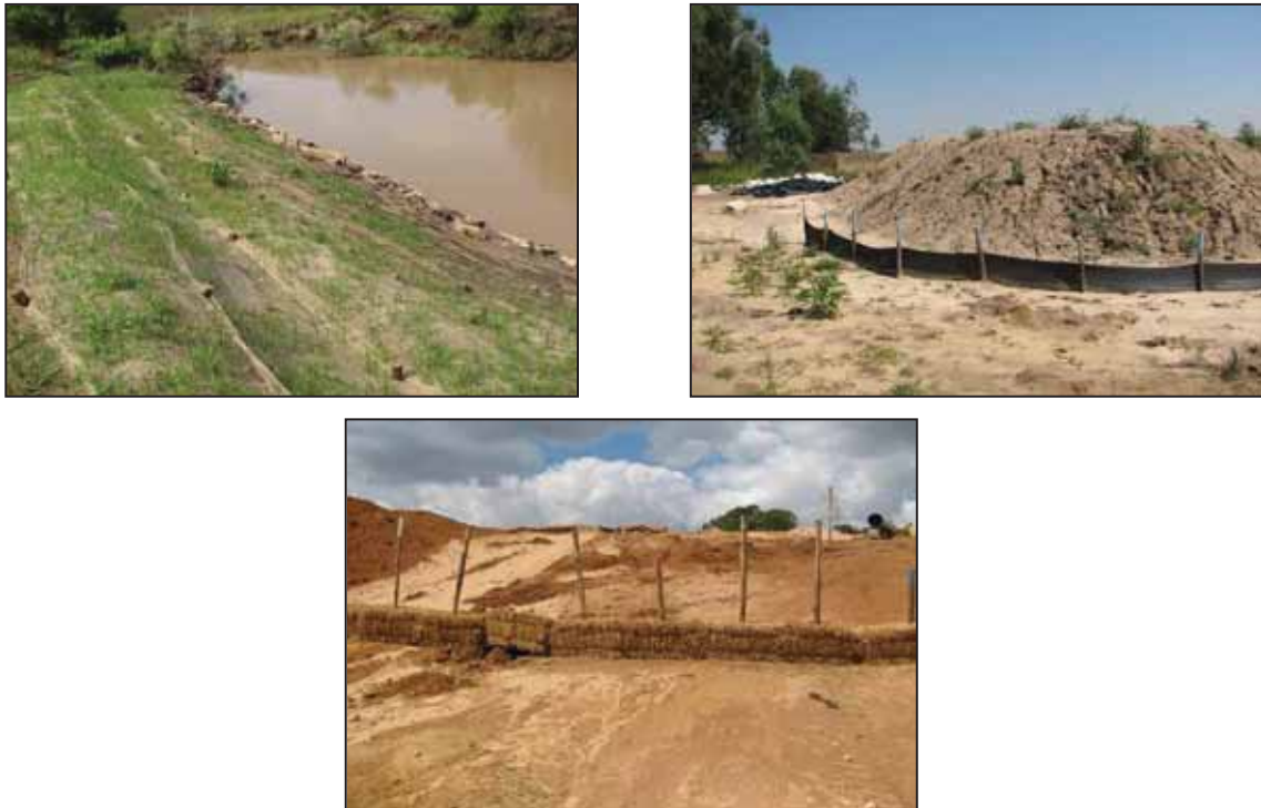
Figure 22: Typical soil erosion mitigatory measure: BioJute Installation ( top left ); a silt fence protecting a stockpile ( top right ) and pegged hay bale wall used to reduce runoff velocities ( bottom )
