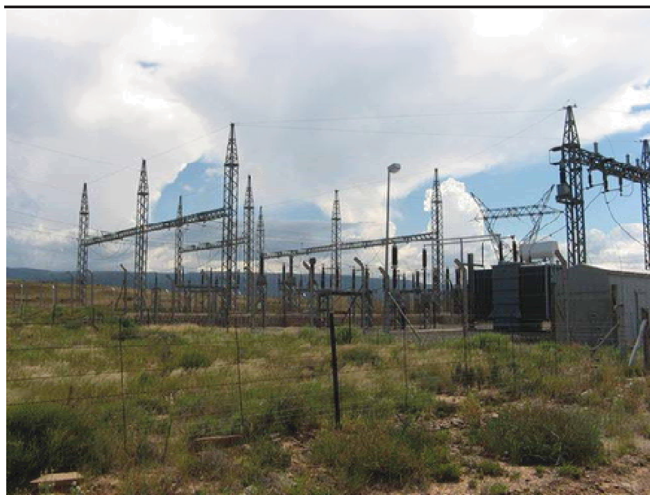
Figure 1.10 Existing Drennan Traction Substation
