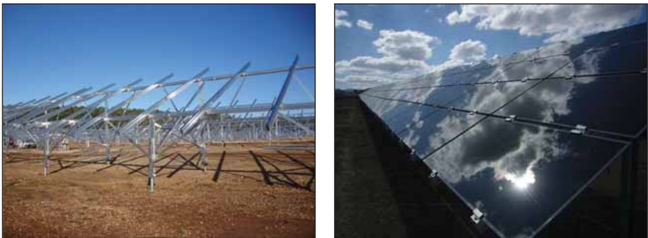
Figure 2: PV Frames and panel arrays (Source: Solaire Direct and ERM, 2012)
