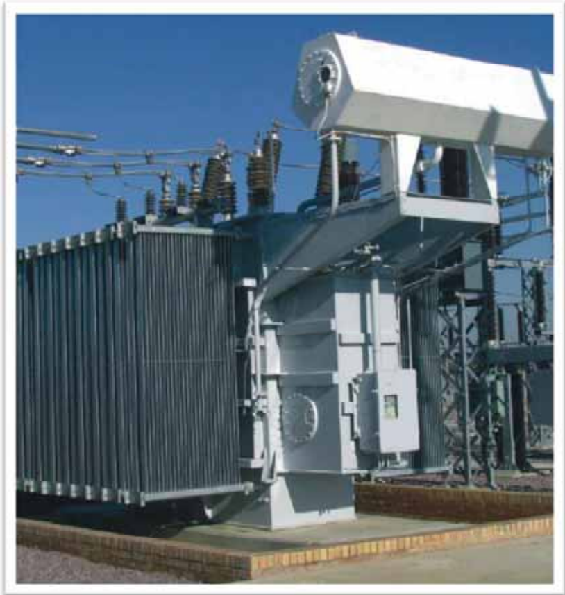
Figure 5: Photograph of proposed power transformer (EMP.2013)
