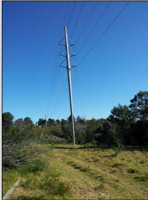
Figure 2: Guyed suspension Tower
