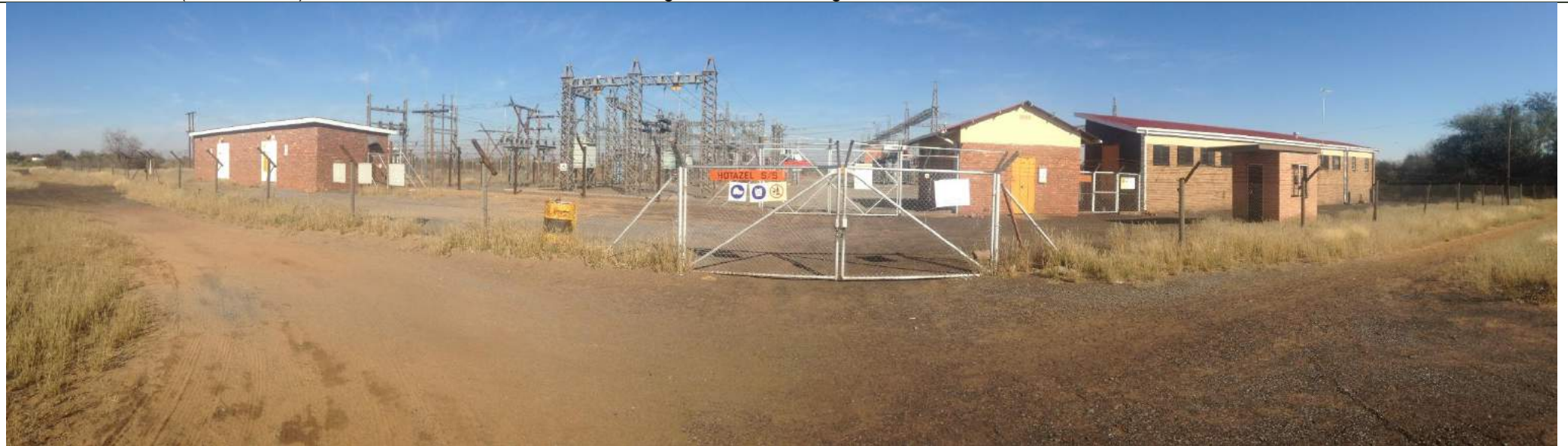
The existing Hotazel substation to which preferred Alternative 1 will connect
