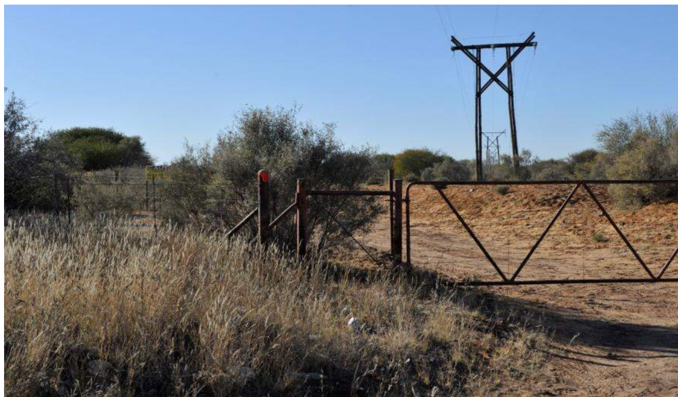
Figure 6: The Hotazel-Riries 66kV line which bisects the area just south-west of the proposed solar area.
