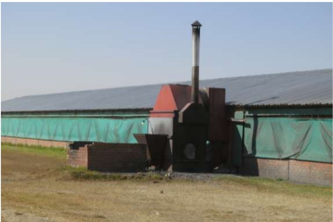
Figure 8: Photograph of a coal fired heater at the existing facility (2).
