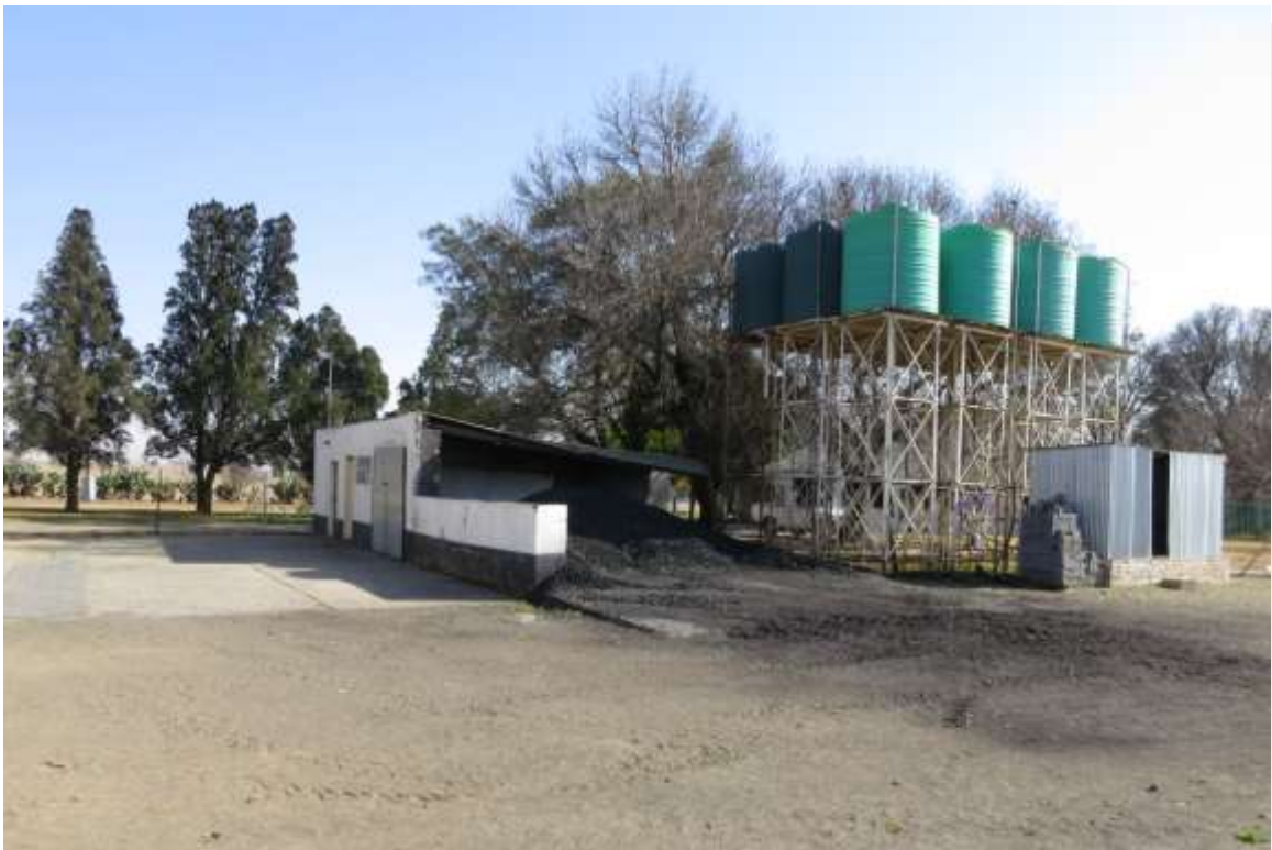
Figure 6: Photograph of the coal storage area and JoJo tanks at the existing broiler facility.
