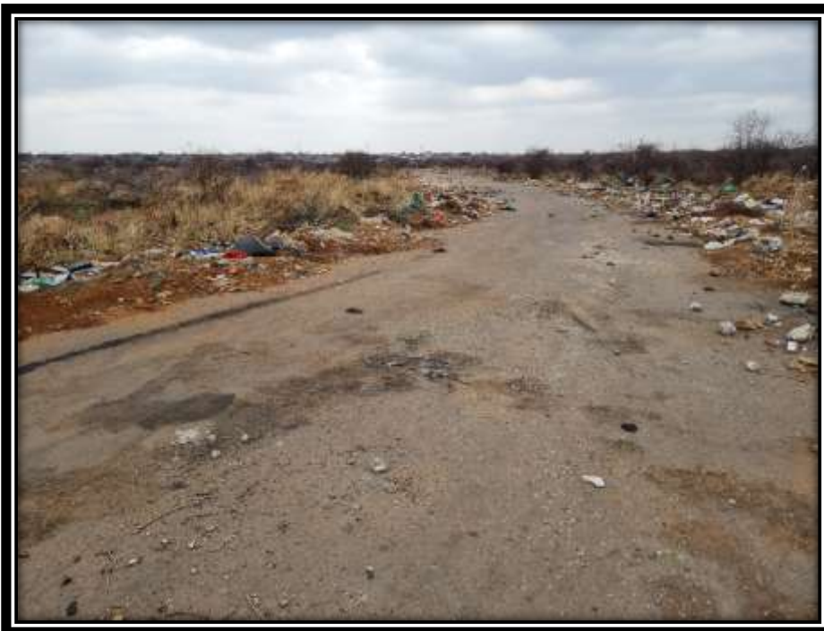
Photograph 6: Old roads run through the site. Once again also note the extensive informal dumping.
