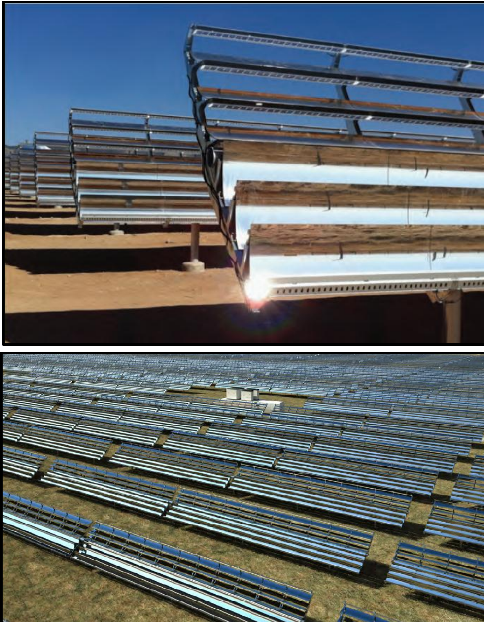
Figure 2.4 C7 Tracker System™ for Forzando North
