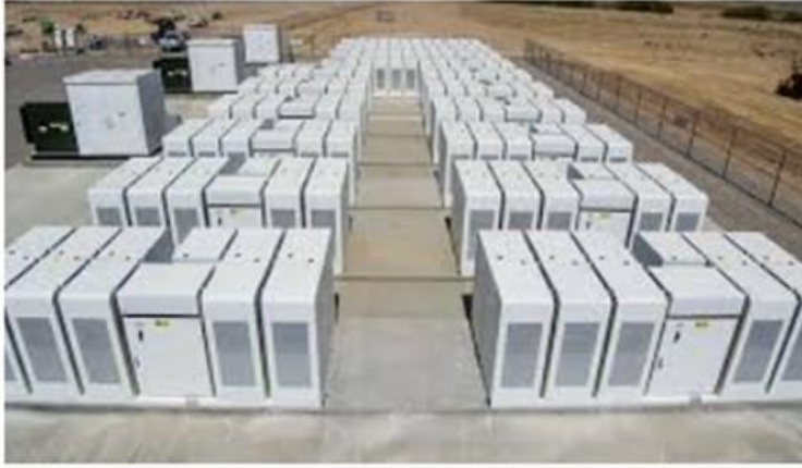
Figure 12: Typical Battery Storage Facility ( www.spglobal.com )
