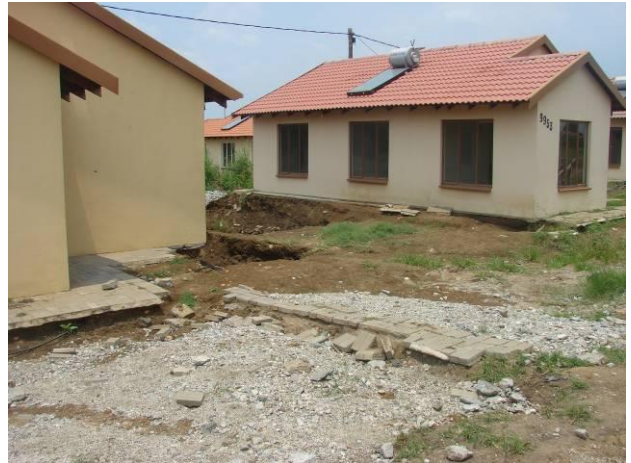
Photo 31 Flooded house taken 2011 /02/02
