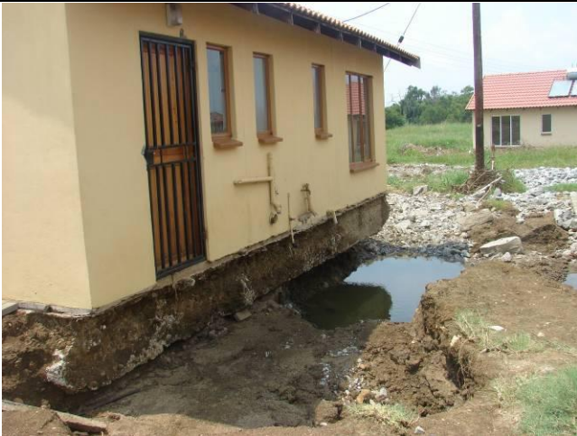
Photo 30 Flooded house taken 2011 /02/02
