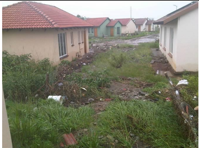
Photo 33 Flooded house taken 2011 /01 /18
