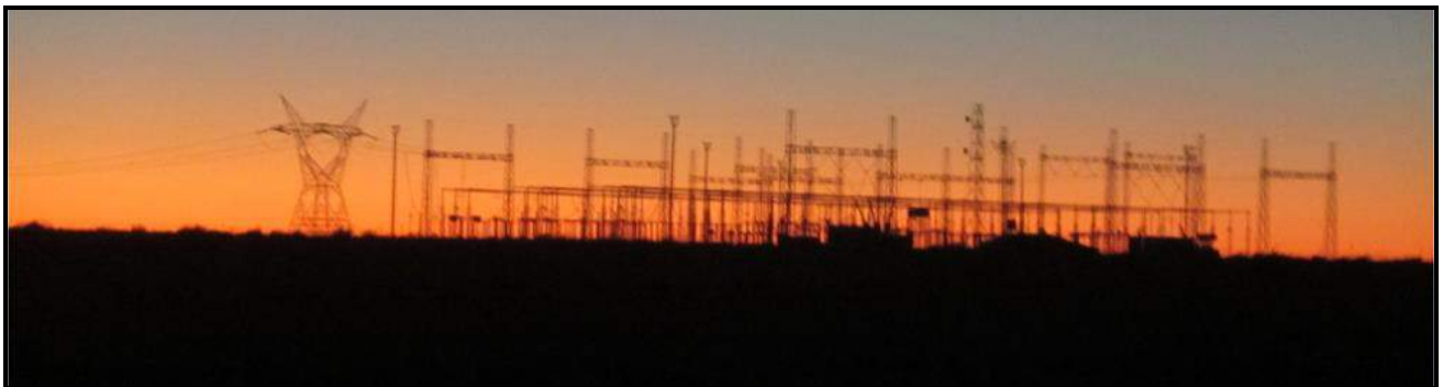
Figure 25: Evening view of the large Eskom substation located some 16 km south of the proposed project.
