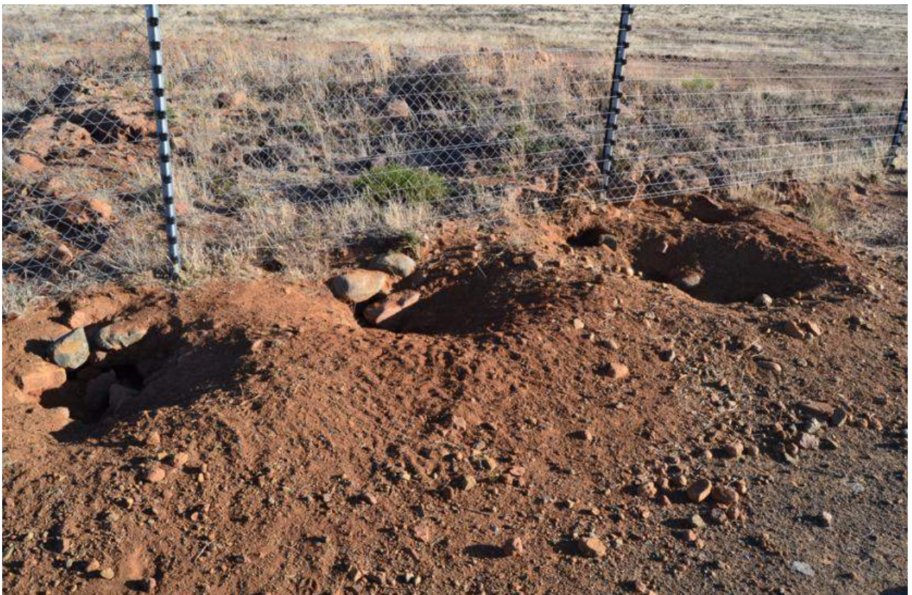
Figure 21: Excavation and movement under fences by larger animals, porcupines and Aardvark ( Orycteropus afer ).
