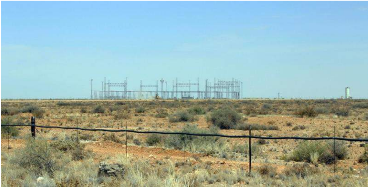
Figure 6: Photograph depicting the Eskom Nieuwehoop substation under construction (CSIR, 2016a; photo credit: Henry Holland).
